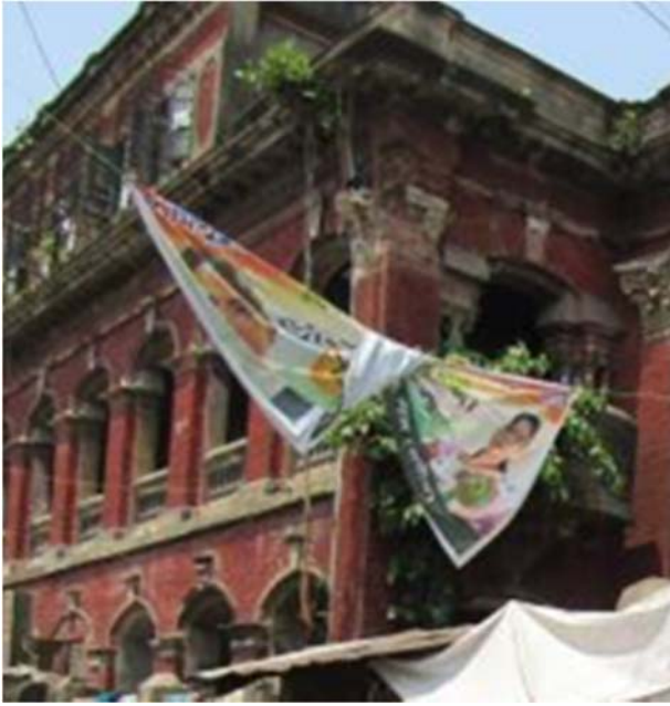
Figure 12. Example of lack of maintenance of advertisements
